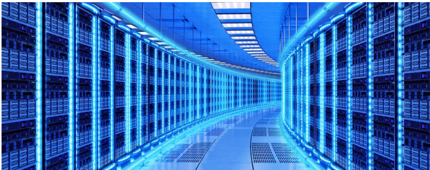
Source: Amazon. Data Centres form the critical infrastructure backbone of Amazon Web Services. These vast storage and computing centres are responsible for generating more than $80bn in revenue annually for Amazon and only a handful of companies are able to deploy globally at the scale that AWS does.
